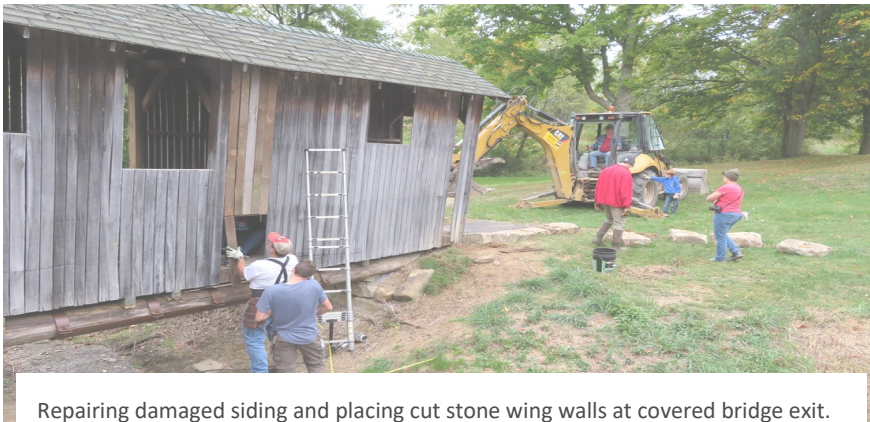
Repairing damaged siding and placing cut stone wing walls at covered bridge exit.
